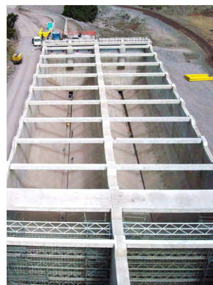
Desander with an integrated flushing device. Project: La Higuera HPP in the Chilean Andes.
