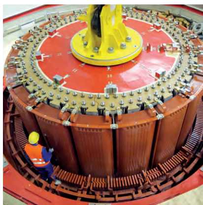
Pumped-Storage Hydropower Plant Vianden, Luxembourg
