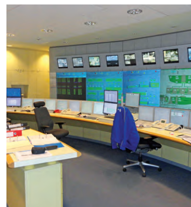
Hydropower Plant Goldisthal, Germany
