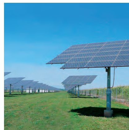
Photovoltaic Power Plant El Palau, Spain
